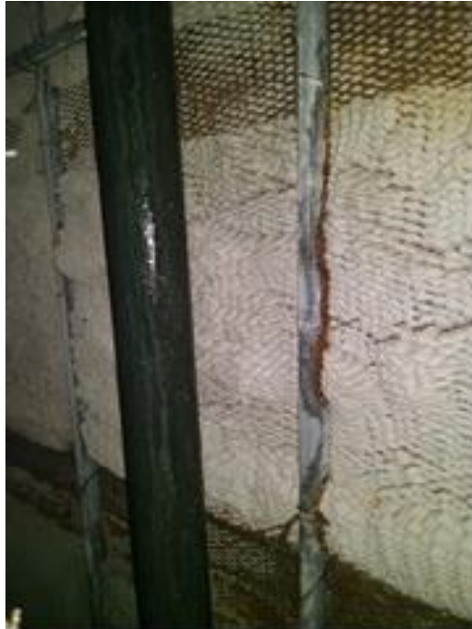
Missing insulation on cold water riser
