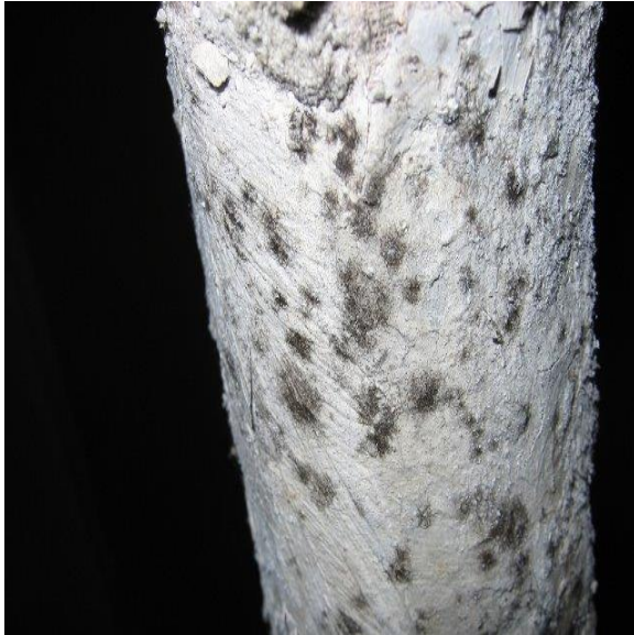
ACM- Pipe insulation (T.S.I)
