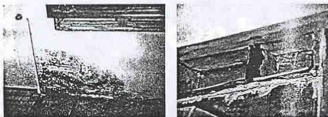
Figure 1. Walls contaminated with a black, slimy fungus later identified as Stachybotrys .
