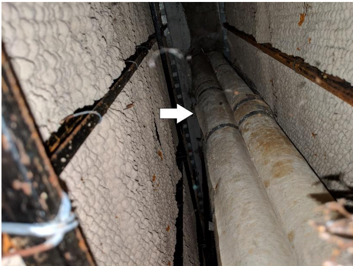
ACM- Pipe insulation (T.S.I)
